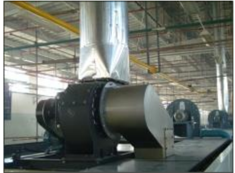
Extraction fan on a DGF oven
